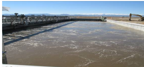
The Aeration Basins are the heart of the treatment process.
